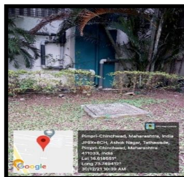
Ground water recharge system
