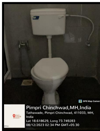
Disabled friendly Toilet
